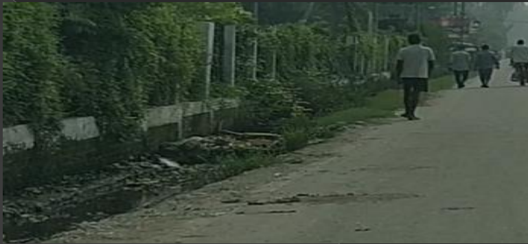
Figure 1: Shoulder drop with water logging and pedestrians moving on road
